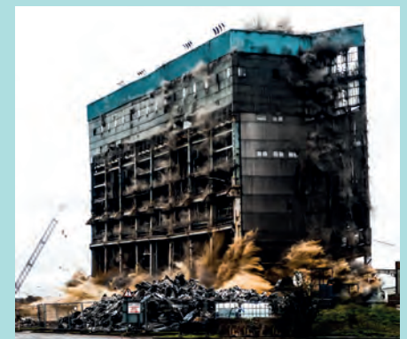
Brown and Mason is one of the world’s leading demolition companies and has an in-house explosive engineering team
