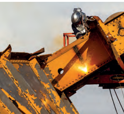
Erith Contractors demolished the turbine hall at Hinkley Point A power station in the United Kingdom
